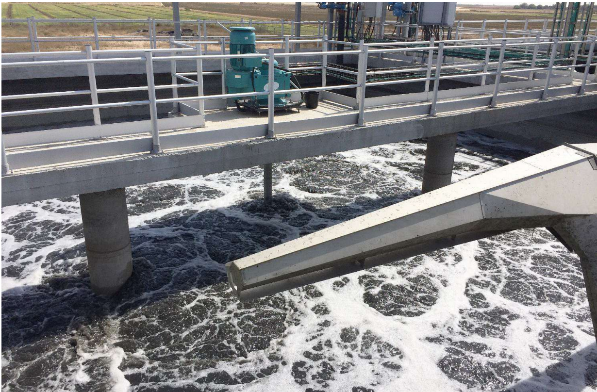
Figure 1: Municipal wastewater treatment plant in Israel with iSBR ®
