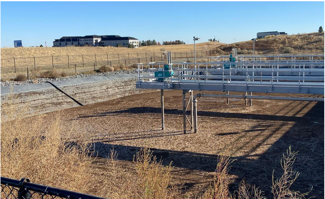
Figure 5: wwtp Meridian, Colorado
